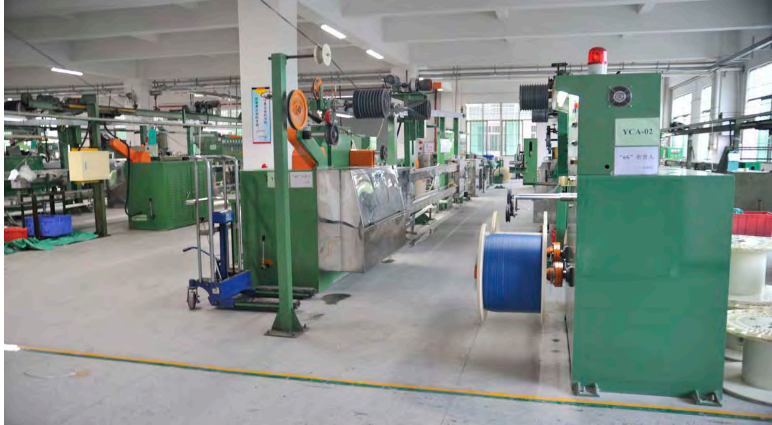
Cable Extrusion Area
